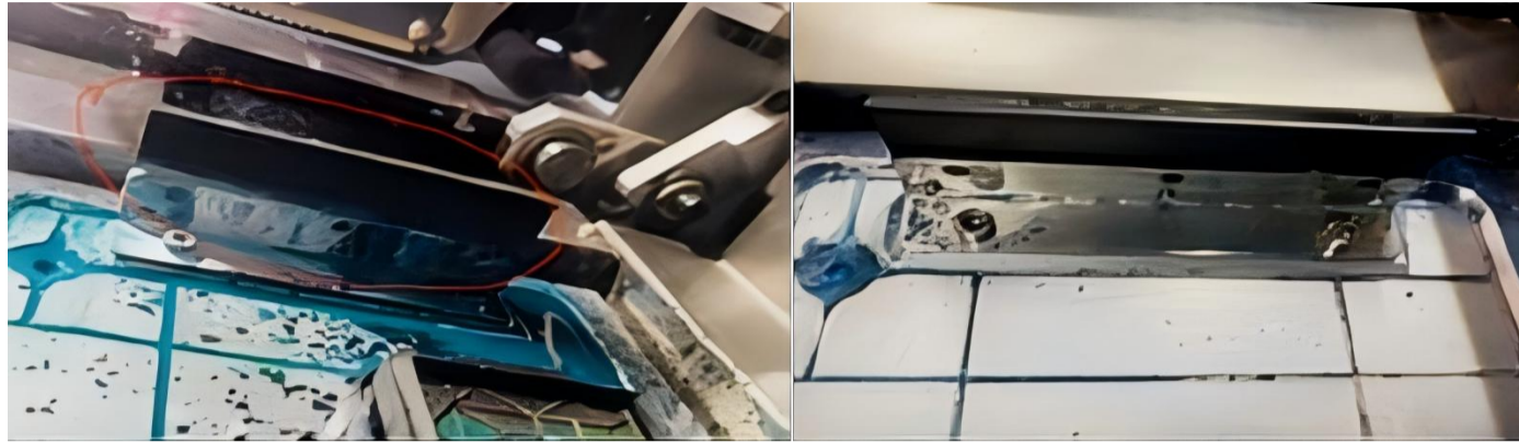
清理前 (Before cleaning)
