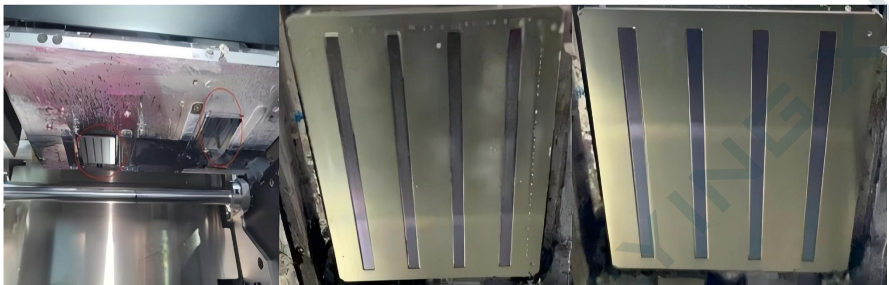
清理前 (Before cleaning)
