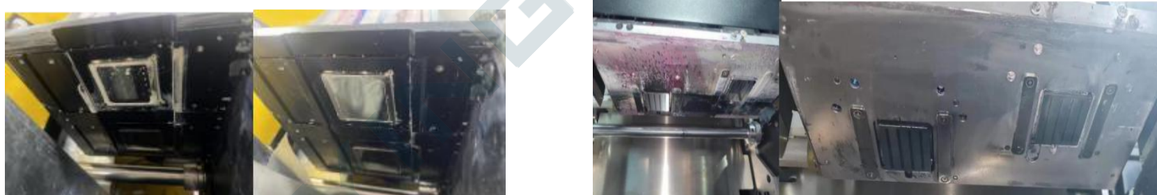
清理前 (Before cleaning)
